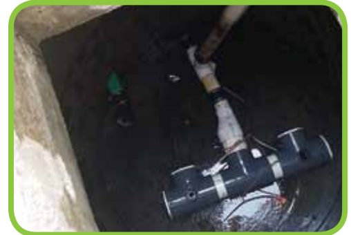
Manifold Tee View of a Cleaned System
