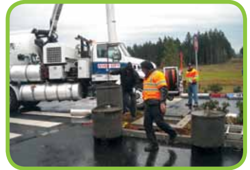
BayFilter System Cleanout
