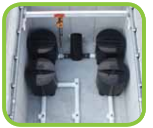
Vault Internal Assembly
