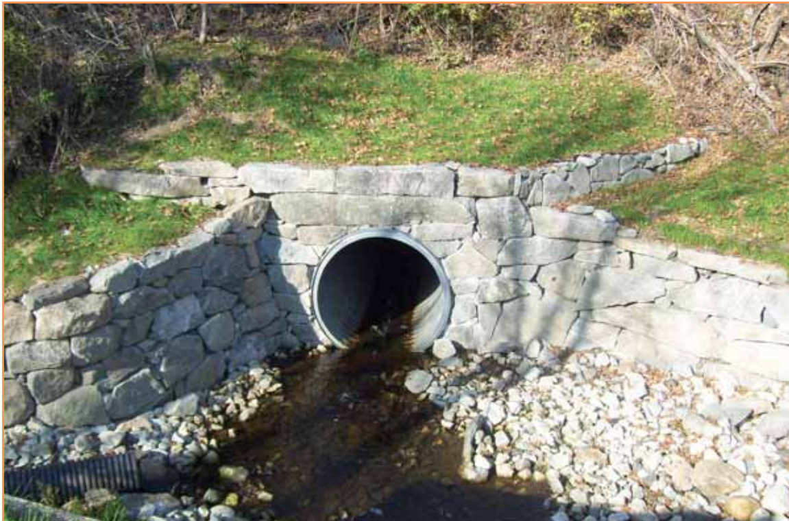
The final headwall and the 60-inch diameter pipe blends in with the surrounding area.
