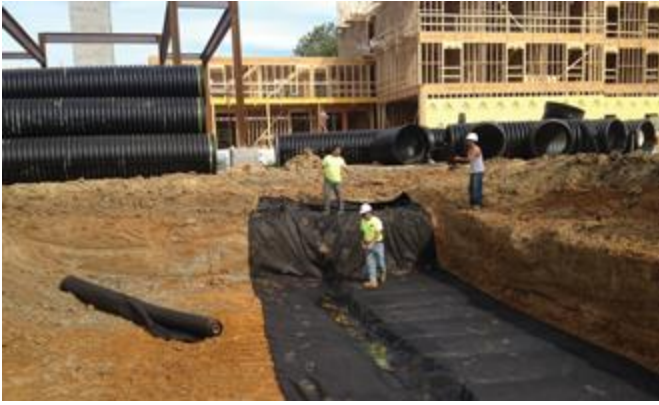
The fabric-wrapped chambers provide for settling and filtration of sediment as stormwater rises in the Isolator Row and ultimately passes through the filter fabric.
