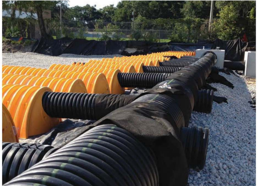
Manifolds for each system were constructed from ADS N-12 corrugated high-density polyethylene pipe.
